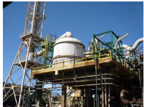
Wet Catalysis Plant filter vessel
