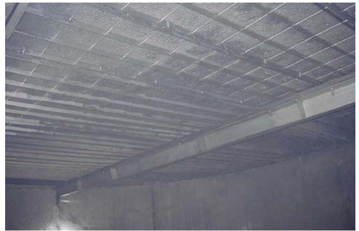
View from below of a Drying Tower Demister
