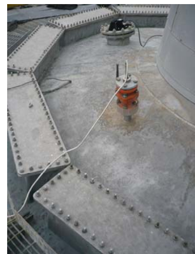
View of Tower Top Demister Panel Access Doors
